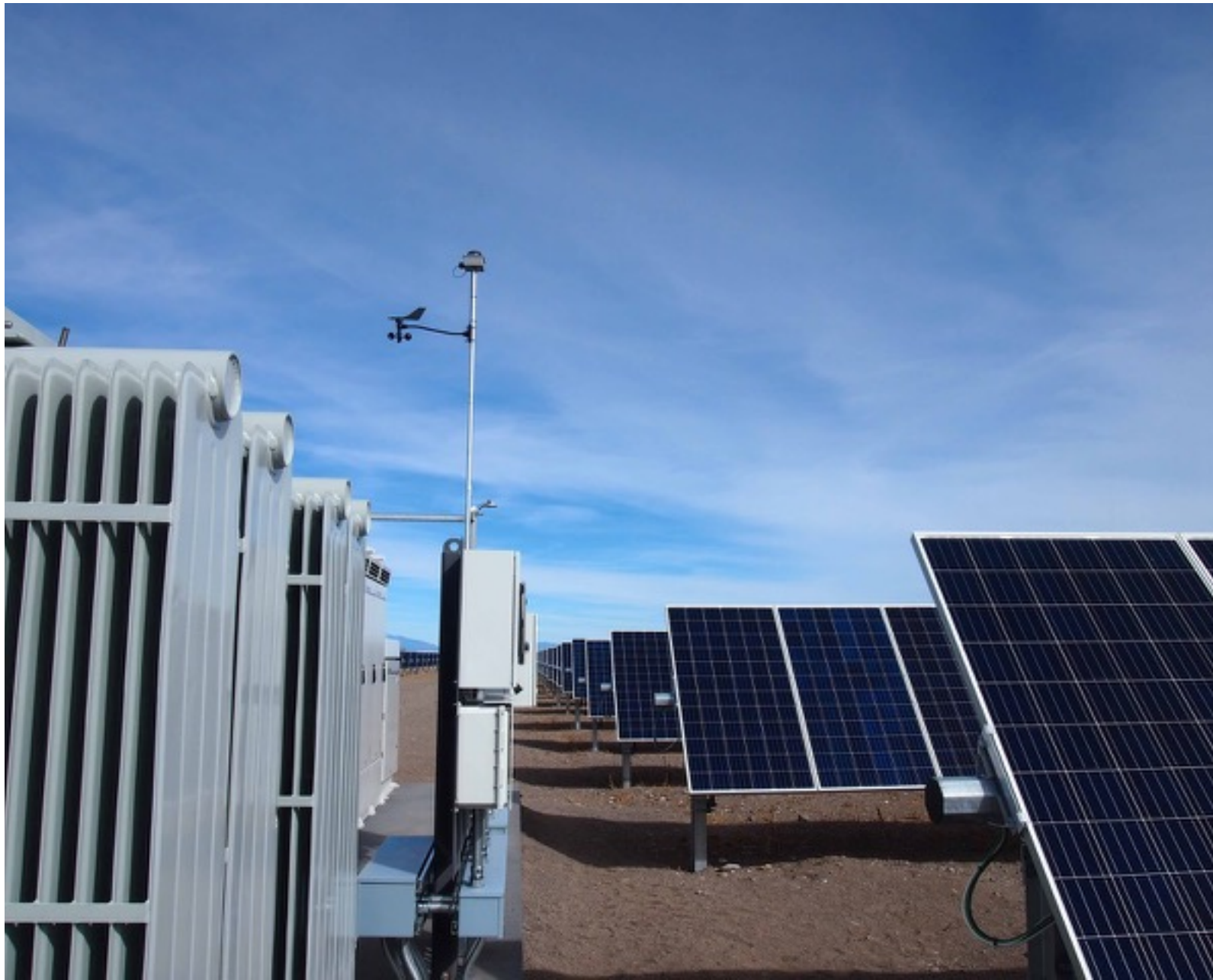
Solar Panels with converter changing Solar Panel DC to AC power. Photo Credit: Rosanne H. Pitcher courtesy of Wolf Creek Ski Area.
