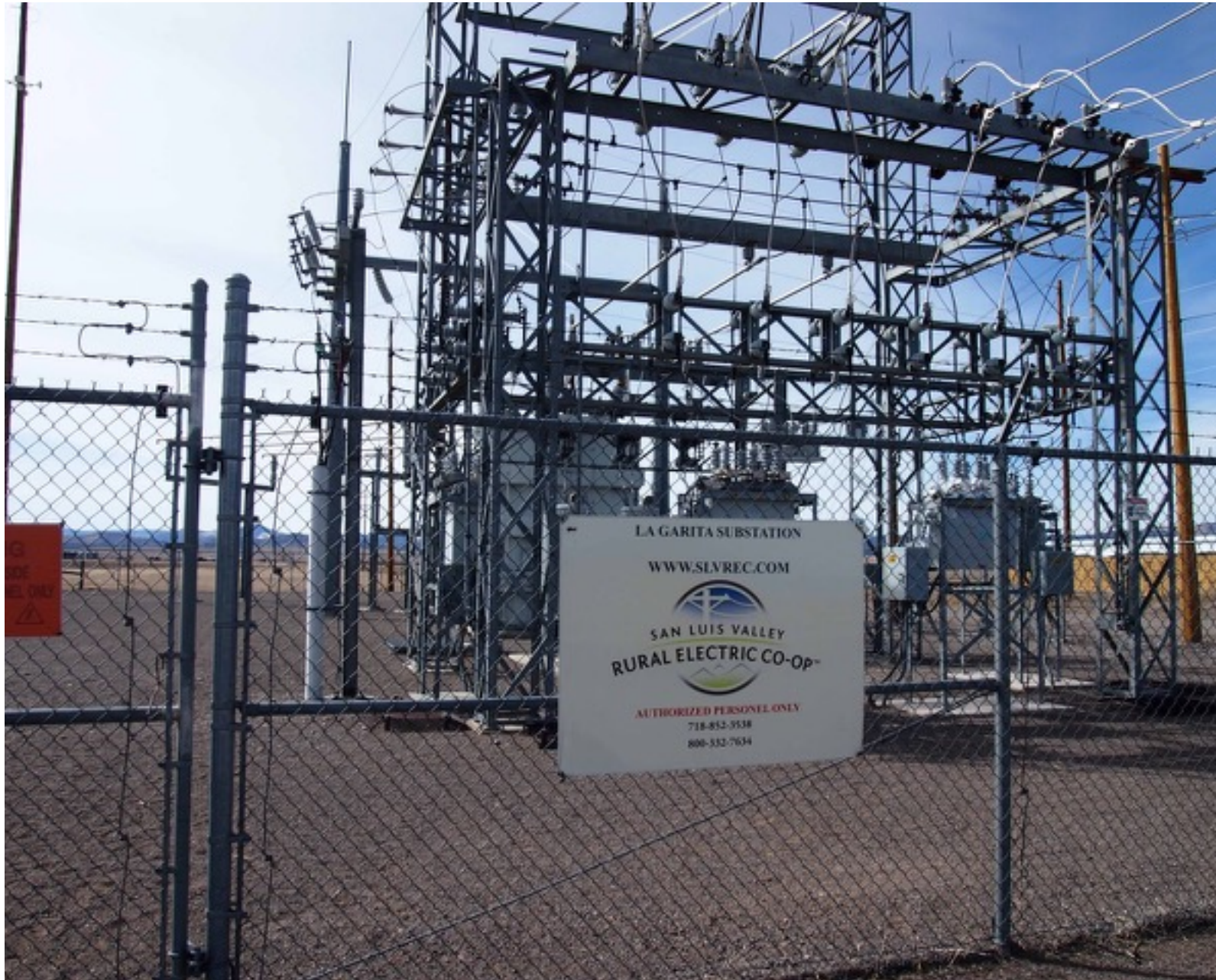
La Garita Substation. Photo Credit: Rosanne H. Pitcher courtesy of Wolf Creek Ski Area.
